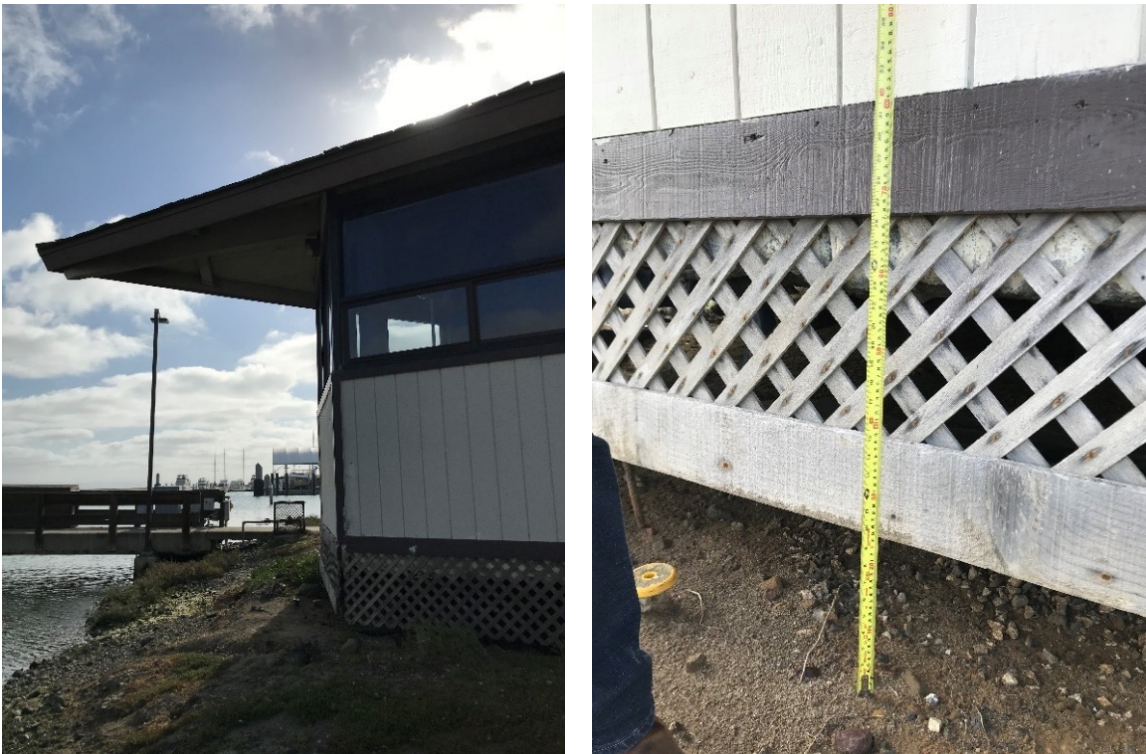
Figure 22. Oyster Point Marina – Harbormaster Building Undermined Foundation (with skirt), 2021
