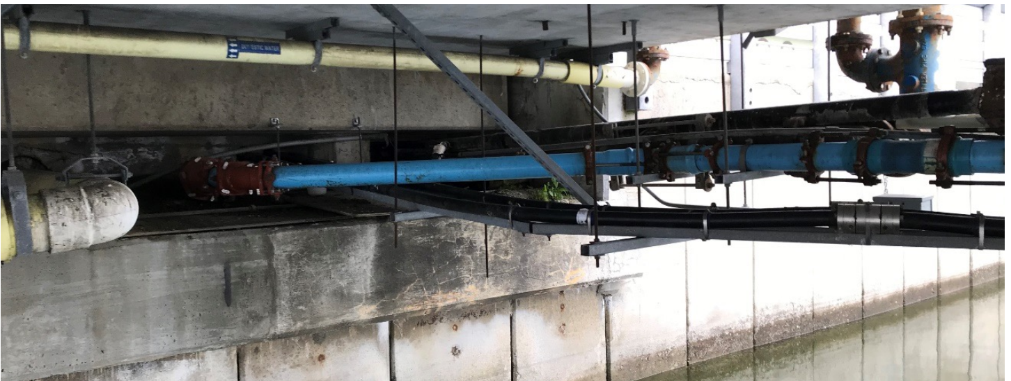
Figure 13. Johnson Pier, Under-deck Utilities at Bulkhead, 2021
