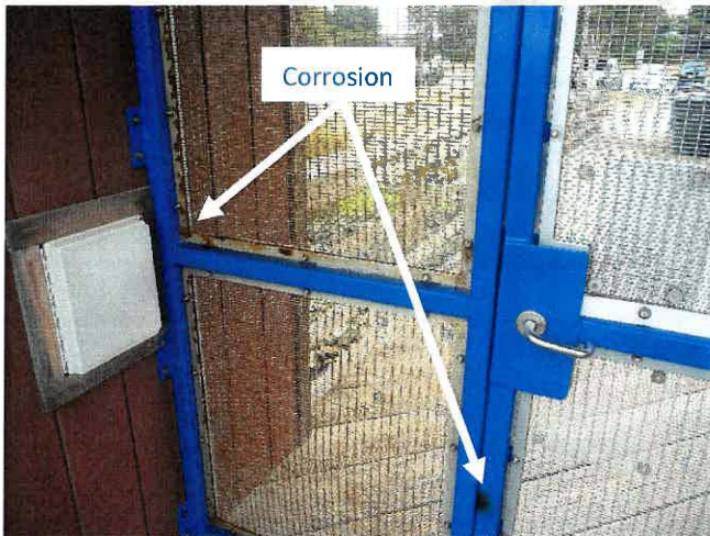
Photograph 16 Typical gate condition with minor corrosion.
