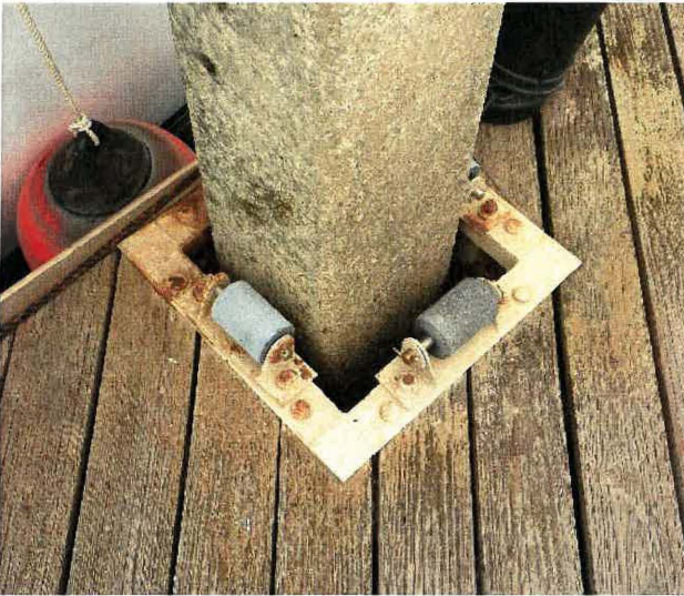
Photograph 4 Pile guide in fair condition, requiring repairs to the galvanic coating
