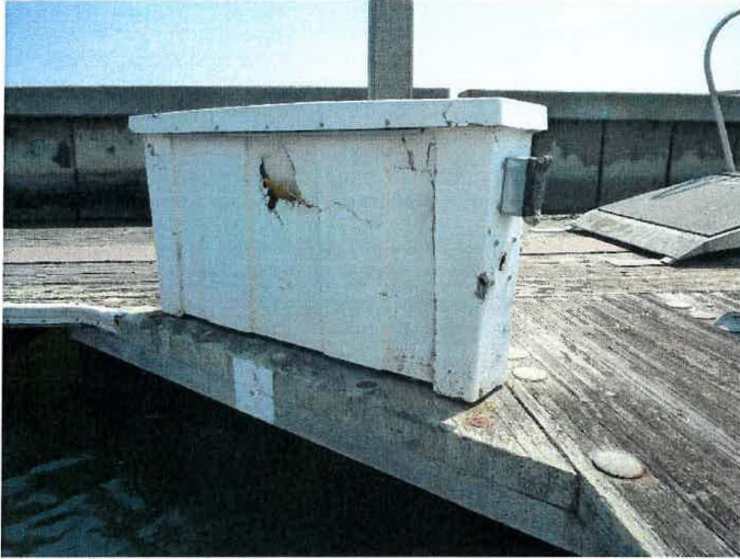
Photograph 21 Broken dock box on Dock 14
