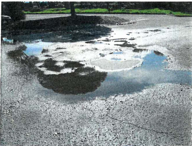
Photograph 9: Potholes & Alligator Cracking
