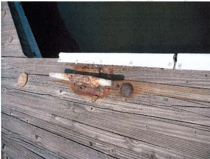
Photograph 9 Cleat in poor condition
