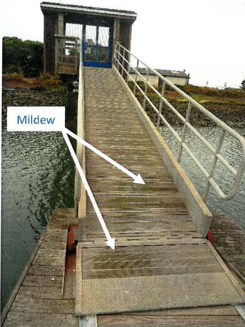
Photograph 15 Typical gangway condition with mildew
