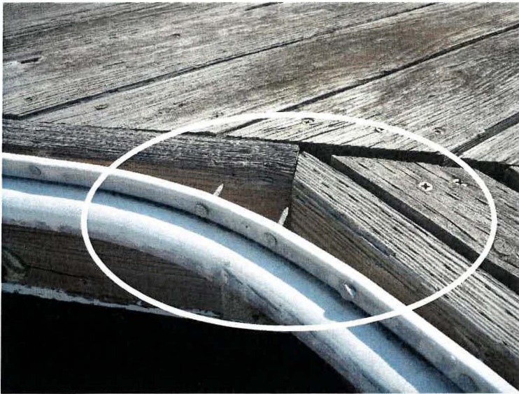
Photograph 6 Detached rub rail with exposed nails
