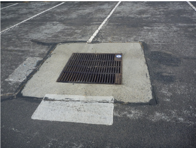
PHOTOGRAPH 15: STORM DRAIN DROP INLET
