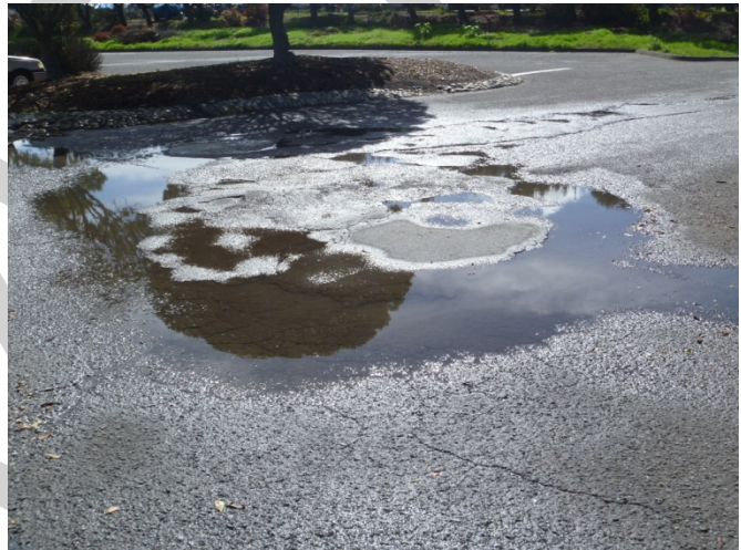
PHOTOGRAPH 9: POTHoles & ALLIGATOR CRACKING
