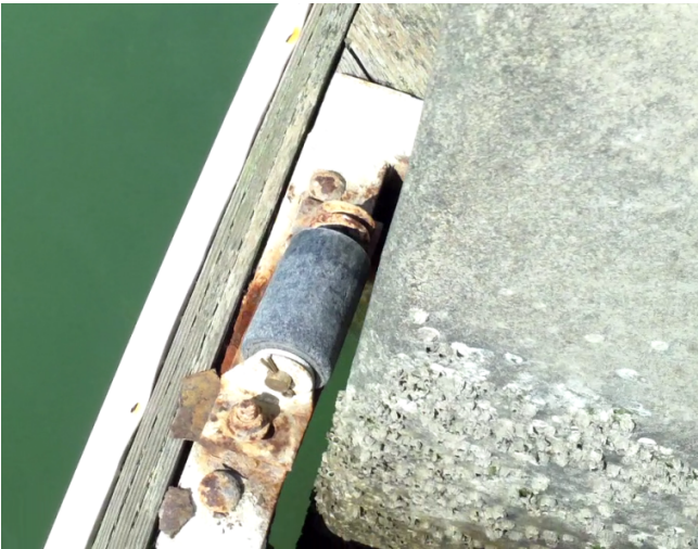
PHOTOGRAPH 2: PILE GUIDE DAMAGE – DOCK 1, SLIP 6-8
