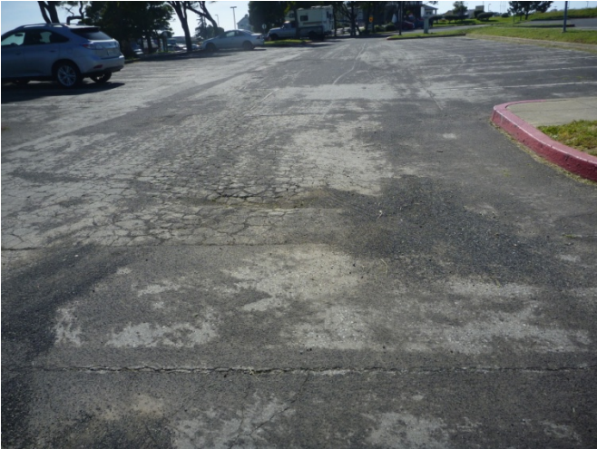
PHOTOGRAPH 14: ALLIGATOR CRACKING NORTH PARKING LOT
