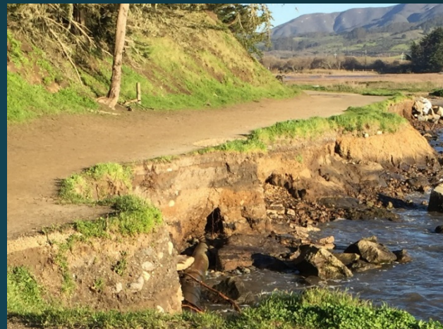
West Trail Erosion Protection
