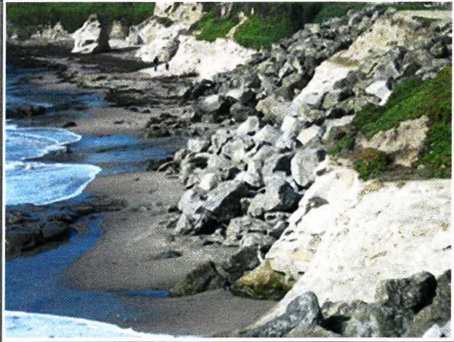
Rip-rap revetments have been installed as coastal protective structures in many locations in Santa Cruz
