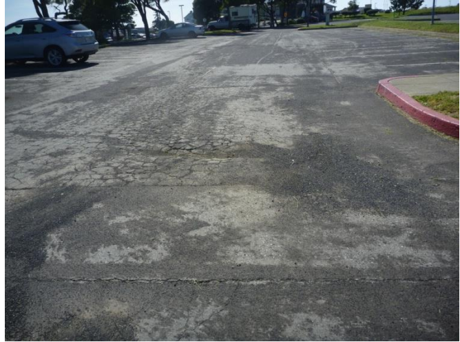
Photograph 14: Alligator Cracking North Parking Lot
