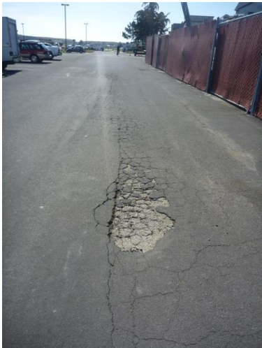
Photograph 13: Potholes & Alligator Cracking West Parking Lot
