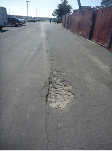
PHOTOGRAPH 13: POTHOLES & ALLIGATOR CRACKING WEST PARKING LOT
