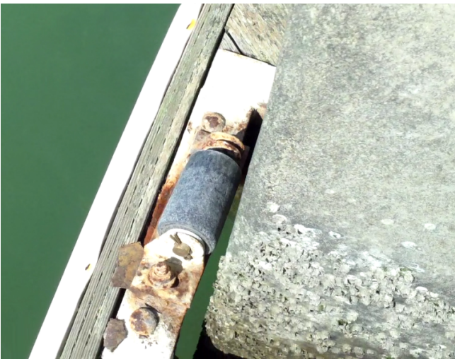
PHOTOGRAPH 2: PILE GUIDE DAMAGE – DOCK 1, SLIP 6-8
