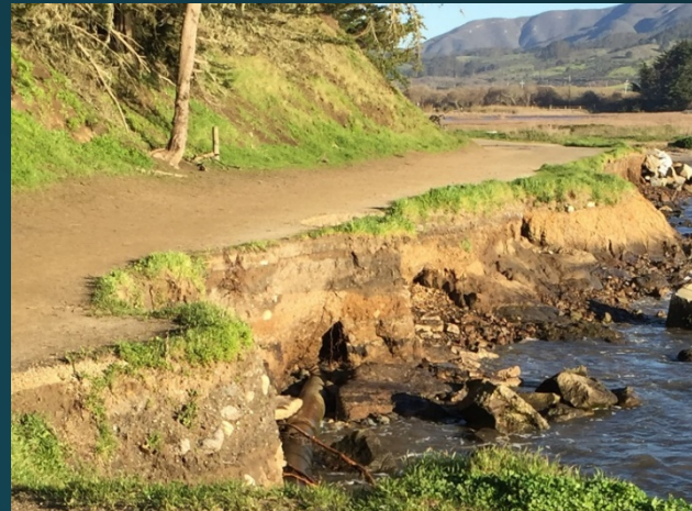
West Trail Erosion Protection
